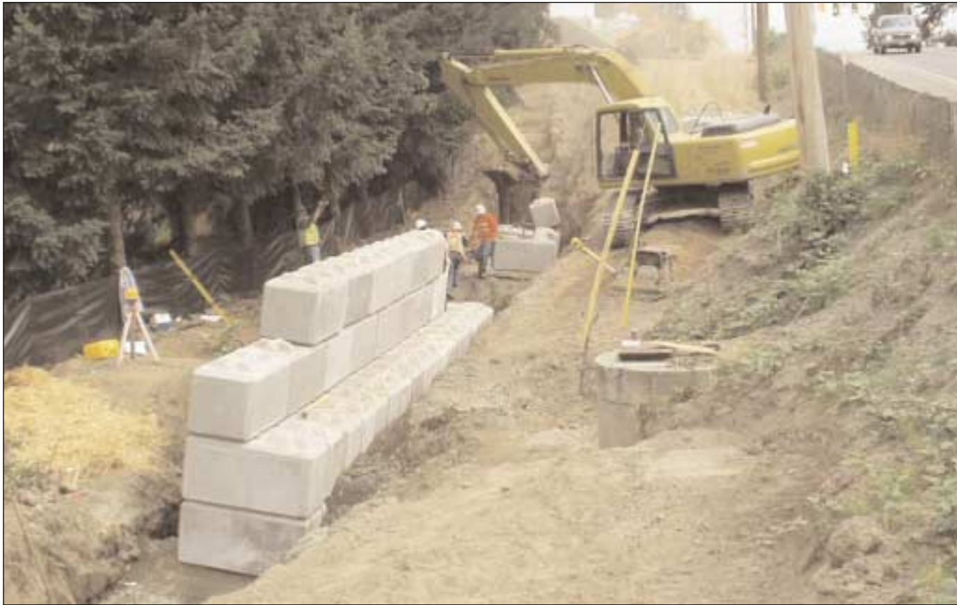
Contractor installing segmental block wall on north side of SE 256th Street
