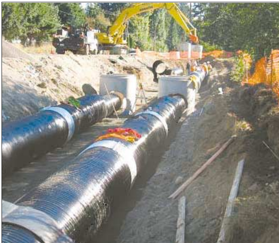
Contractor installing 48-inch diameter asphalt-coated and galvanized corrugated metal storm detention pipes and control structure manholes.
